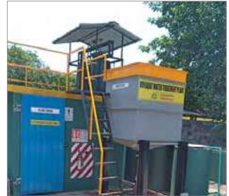
Effluent treatment plant at Jaffna workshop
