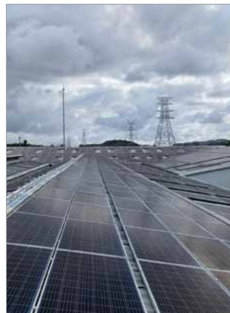
Ratmalana Roof top Solar Installation
